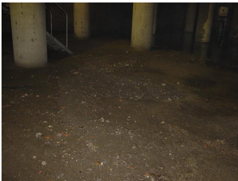
Fig. 1. Sedimentation in storm tank.
